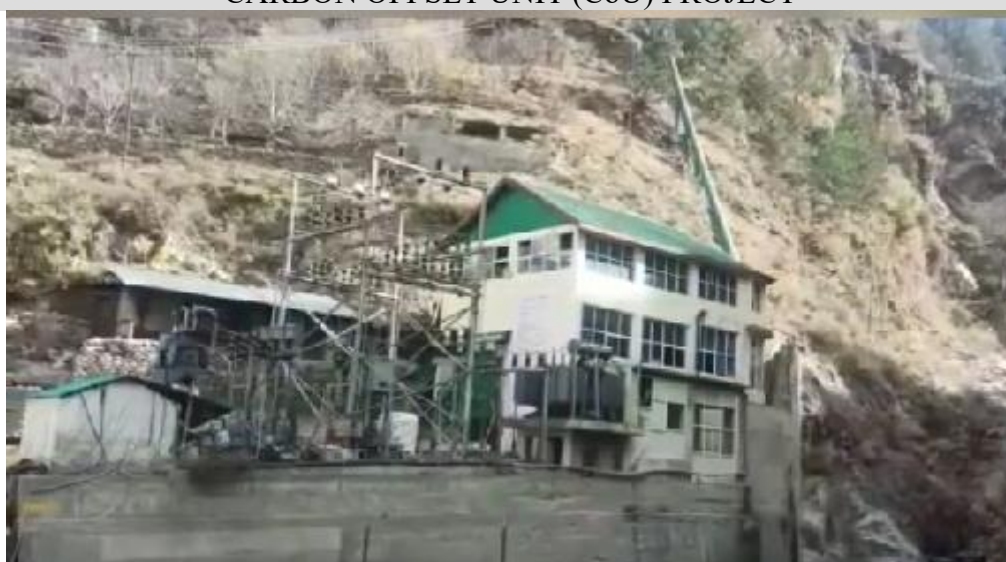
3 MW Shyang Small Hydro Electric Project
